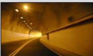
Lighting of tunnels
