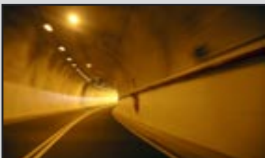
Lighting of tunnels
