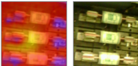
Detect issues with switchgears
