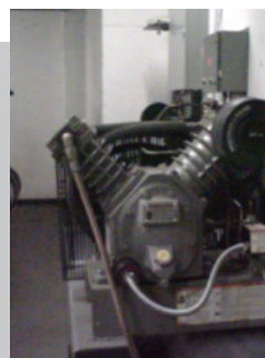
Air Compressor – Full Visible
